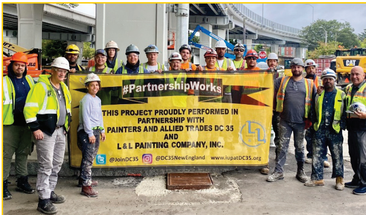
L&L Painting Crew working at the Chelsea Viaduct, including Amanda Rivera, Superintendent Mark Burdick, Luis López, Robrer Montes, Adriano Knupp, Pablo Ruiz, Jesse Monteiro, Phyllis Desmings, Paul Neves, Francisco Santiago, Valerio Cardoso and Tyler Laporte.
