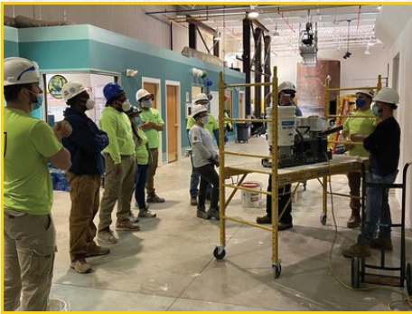
Apprentice Drywall Finishers learn the use and application of No Coat beads and trims.
