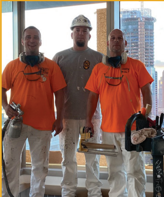
Right to left: performing the window mullions repairs are Mike Lasota, DC 35 Steward; John Dowd; and Corey Chaggaris.
