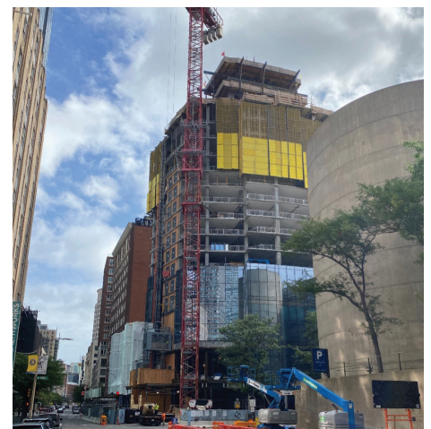
The Raffles Project at 40 Trinity Place in Boston is finally rising out of the ground. Cheviot Corp has the unitized curtain wall.
