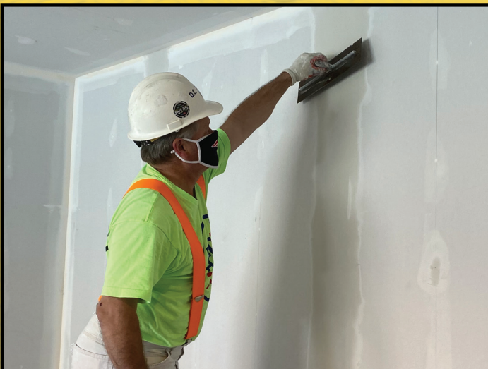
DC 35 Steward Steve Bettencourt applying the drywall finish at the Edwina Martin House charity job.
