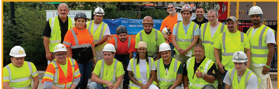
AFL-CIO Housing Investment Trust Fund at work at Old Colony, phase three. DC 35 members are working on site for M. L. McDonald Paint Co. and International Finish Systems.
